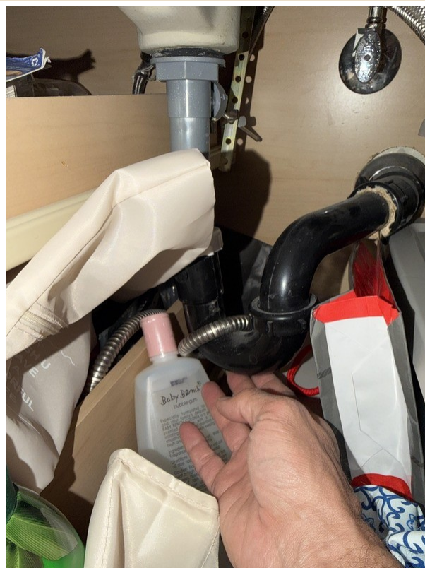
Under-sink plumbing — no leaks
