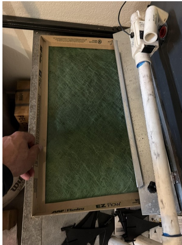
HVAC filter — in service
