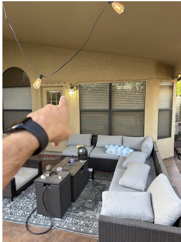
⚠ Patio string lights connected to outlet without GFCI protection
