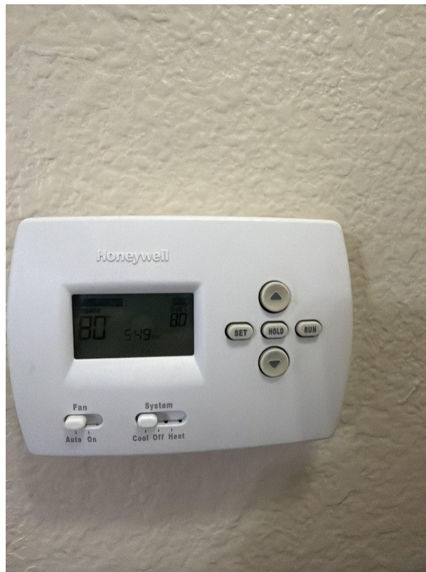
Thermostat — Honeywell, functional
