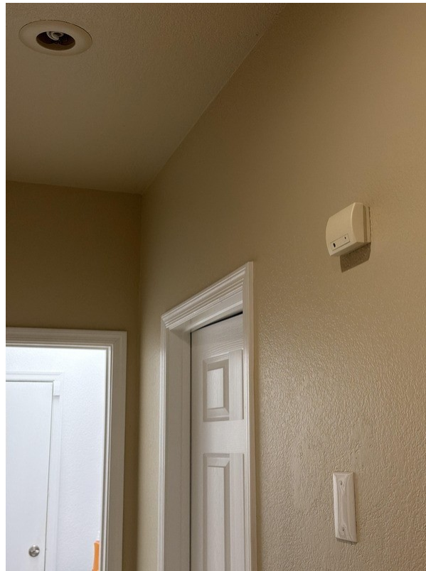
⚠️ Smoke detector — visibly aged unit, requires replacement
